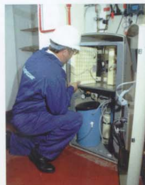
Legionella beater: an installation of Aquazur's Envirox system.
